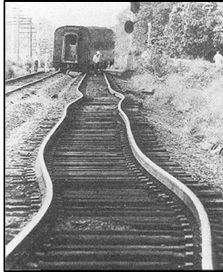
Thermal Expansion of railroad track due to excessive heating. Yes, they would close the track at this point! (Notice the derailed car in the background.)
